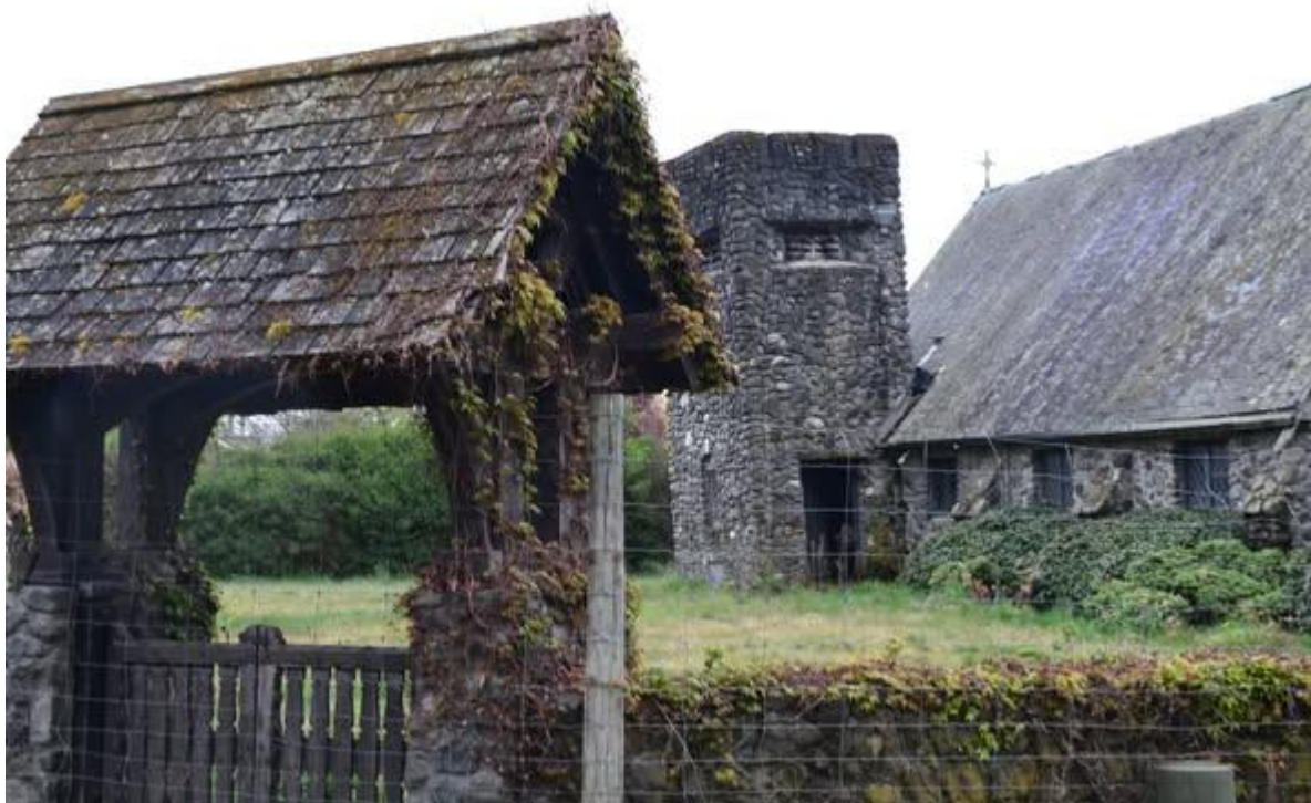
Figure 5. Photograph of All Saints Anglican Church in Waiau showing earthquake-related damage to the building. Photograph taken in October 2025 by Trevor Willetts.
